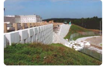
Block retaining wall collapses after heavy rains
